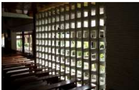
Picture 13 Non-solid wall that was destroyed during the earthquake
