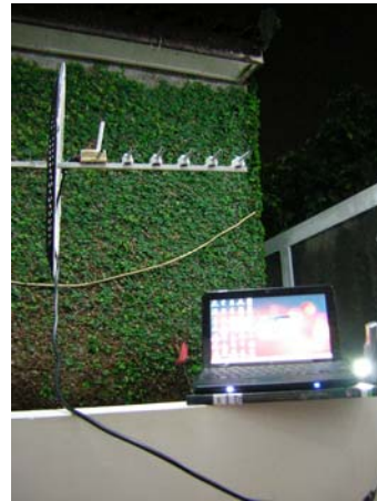
Foto Set-up Antena – Modem – Laptop
