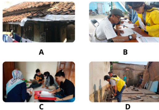
Fig. 3. Identifying damage to the house to control the construction of the house
