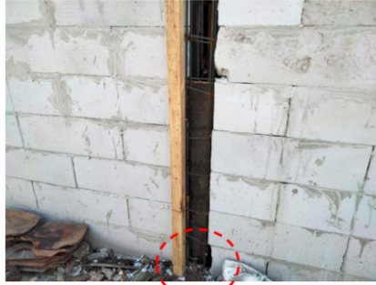
Fig. 13. Sloof is not tied to the foundation
