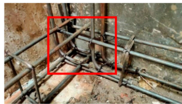
Gambar 26. Kesalahan Detailing Sloof
