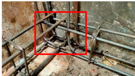
Gambar 26. Kesalahan Detailing Sloof
