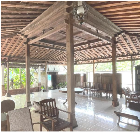
Figure 3. Four main columns (Sokoguru) and main beams (Blandar) as a frame system located in the center of building
