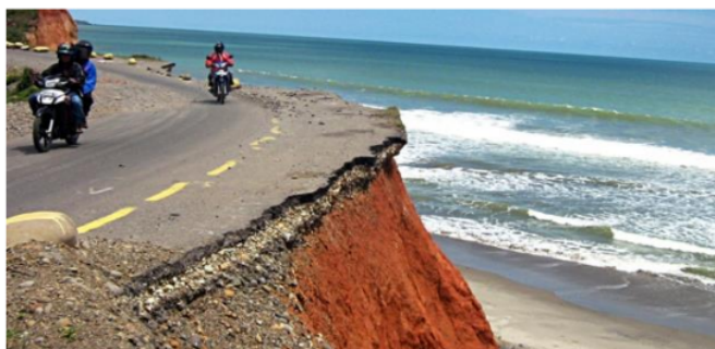
Figure 1. Abrasion at South Kaur District, Kau Regency, Bengkulu Province
