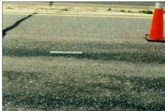
Gambar 2 Jenis Kerusakan Bleeding [British Columbia Ministry of Transportation, 2002]
