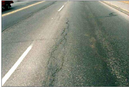
Gambar 7 Jenis Kerusakan Longitudinal Wheel Path Cracking [British Columbia Ministry of Transportation, 2002]
