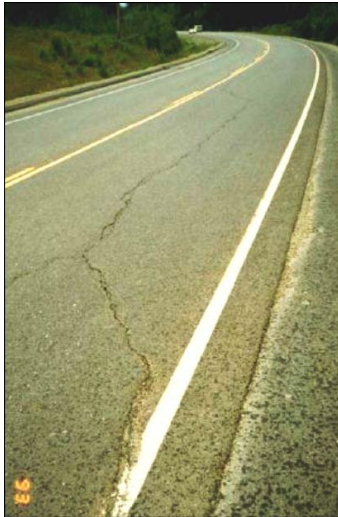
Gambar 16 Jenis Kerusakan Meandering Longitudinal Cracking [British Columbia Ministry of Transportation, 2002]
