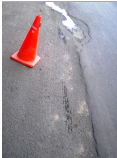
Gambar 14 Jenis Kerusakan Lane/shoulder drop off
