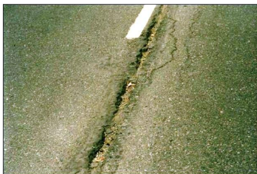
Gambar 6 Jenis Kerusakan Joint Reflection/Longitudinal Joint Cracking [British Columbia Ministry of Transportation, 2002]
