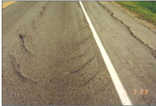
Gambar 10 Jenis Kerusakan Shoving [British Columbia Ministry of Transportation, 2002]
