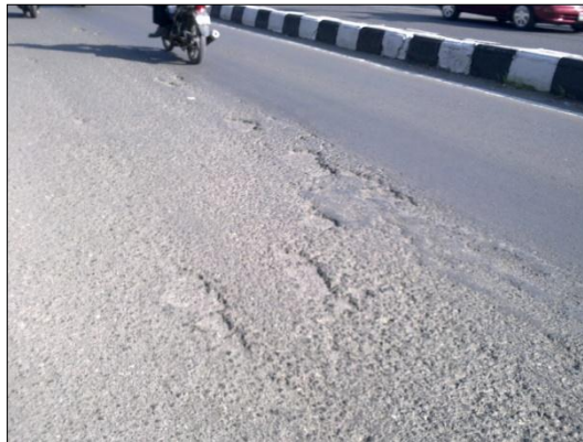
Gambar 11 Jenis Kerusakan Weathering and Raveling
