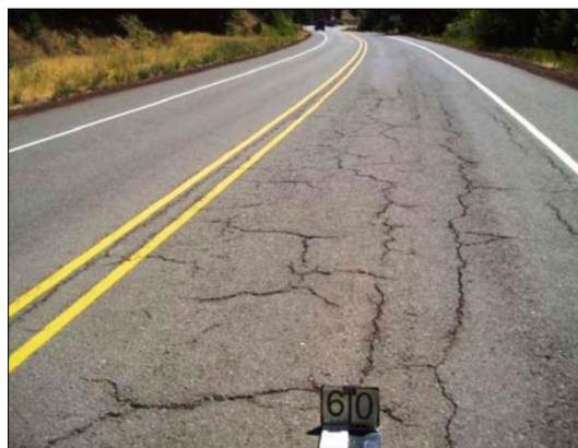
Gambar 3 Jenis Kerusakan Block Cracking [Oregon Department of Transportation, 2010]
