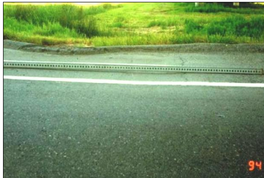
Gambar 5 Jenis Kerusakan Depression/Distorsion [British Columbia Ministry of Transportation, 2002]
