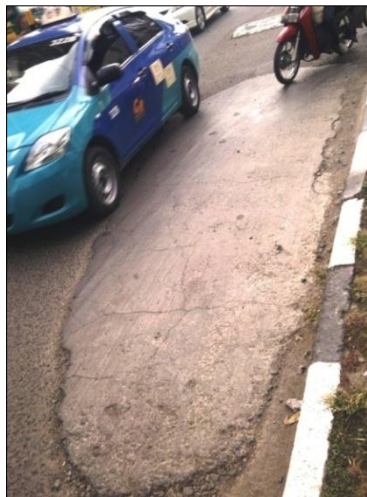
Gambar 17 Jenis Kerusakan Patching and Utility Cut Patching
