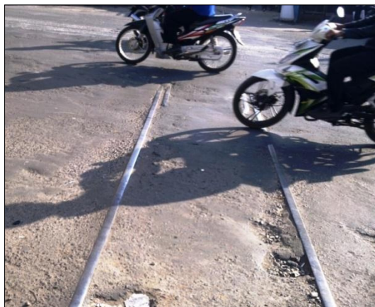
Gambar 9 Jenis Kerusakan Railroad Crossing
