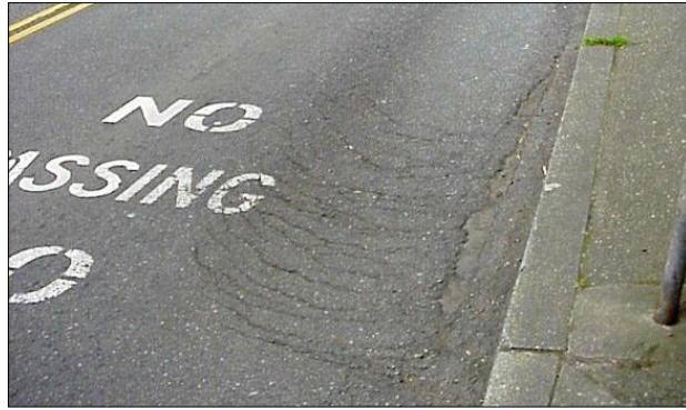
Gambar 13 Jenis Kerusakan Slippage Cracking [Northwest Pavement Management Systems, 1992]
