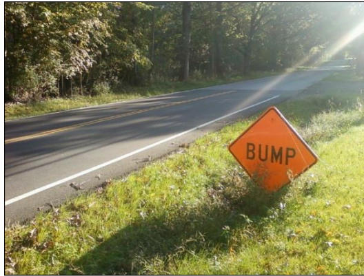
Gambar 4 Jenis Kerusakan Bumps and Sags [Northwest Pavement Management Systems, 1992]
