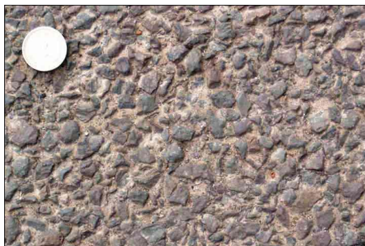
Gambar 12 Jenis Kerusakan Polished Aggregate [Northwest Pavement Management Systems, 1992]
