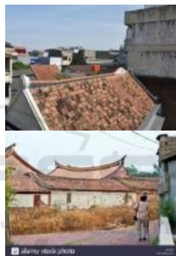
Figure 7: The ending roof ridge is sloping up at both ends, similar with traditional Southern China typical ridge architecture. Here the sloping is with corner and straight line, while the traditional style is smooth arc without any sharp bent.
