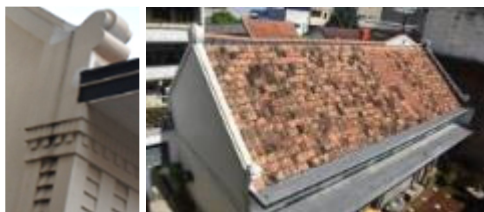
Figure 5: The current roofing and gable wall condition, the 2 ends of gable sloping, finished with curls.
