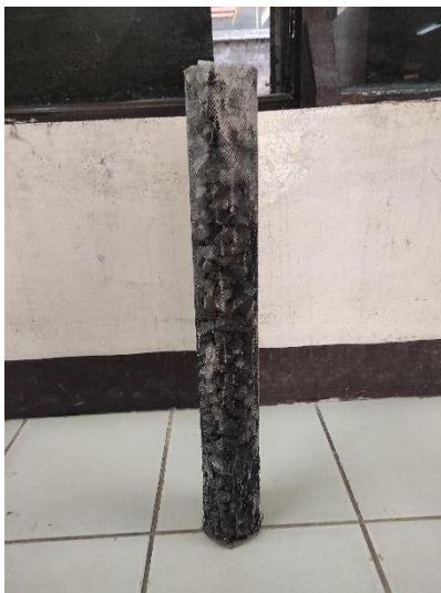
Fig. 2. Porous concrete of bridge pier
