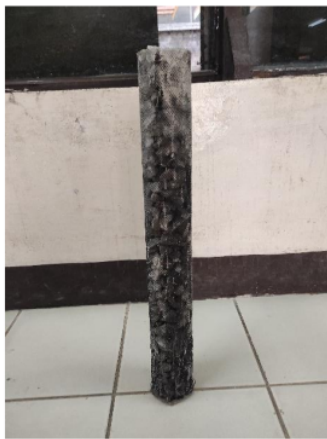
Fig. 2. Porous concrete of bridge pier
