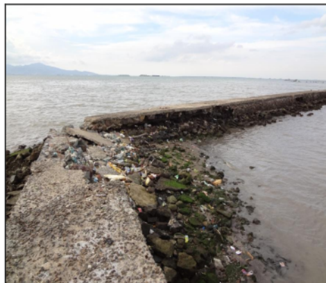
Figure 12 Damage condition on Karangantu's Jetty
