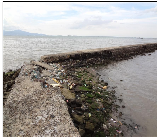
Figure 12: Damage condition on Karangantu's Jetty
