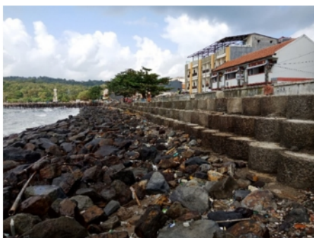
Figure 7: Conditions of Breakwater in the East Coast Pangandaran at Coordinates 07^{\circ} 41' 55,93'' S; 108^{\circ} 39' 33,23'' E.
