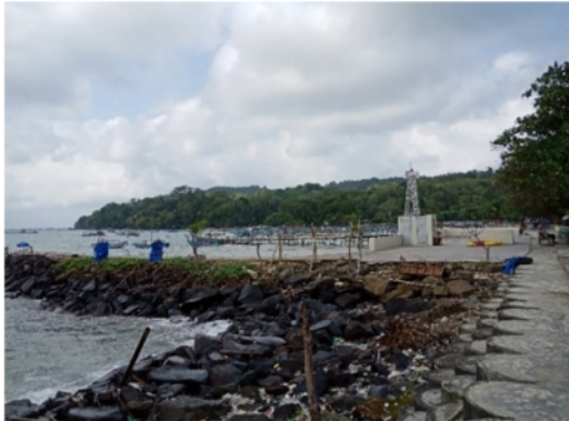
Figure 5: Condition of Breakwater in East Coast Pangandaran at Coordinates 07^{\circ} 41' 55,62'' S; 108^{\circ} 39' 33,20'' E.
