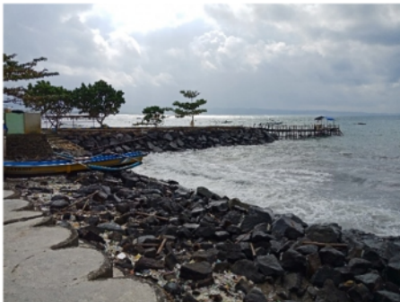
Figure 6: Condition of Breakwater in the East Coast Pangandaran at Coordinates 07^{\circ} 41' 54,69'' S; 108^{\circ} 39' 33,54'' E.
