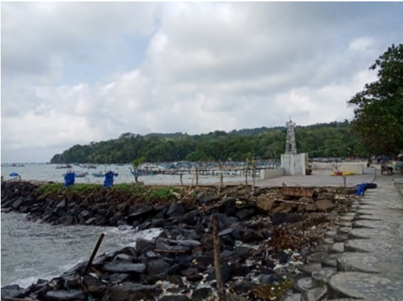
Figure 5: Condition of Breakwater in East Coast Pangandaran at Coordinates 07° 41' 55,62" S; 108° 39' 33,20" E.
