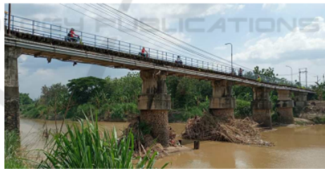
Figure 1: Local scouring around the pier (From: Bintangtimur.net).
