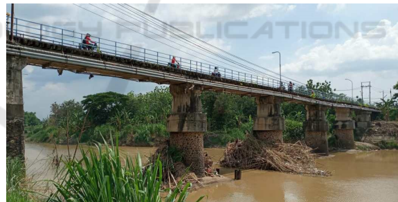
Figure 1: Local scouring around the pier (From: Bintangtimur.net).
